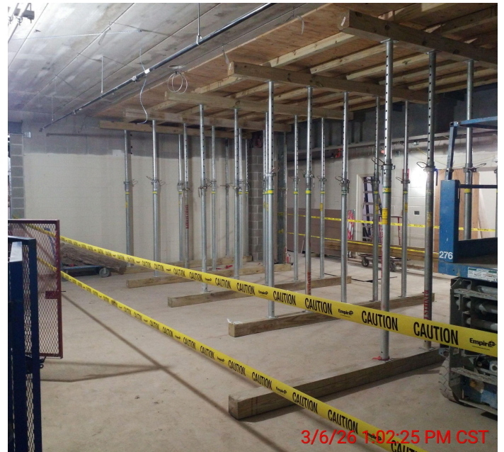
Lower level in former Council Chambers facing SE: bracing to support removal of concrete above
