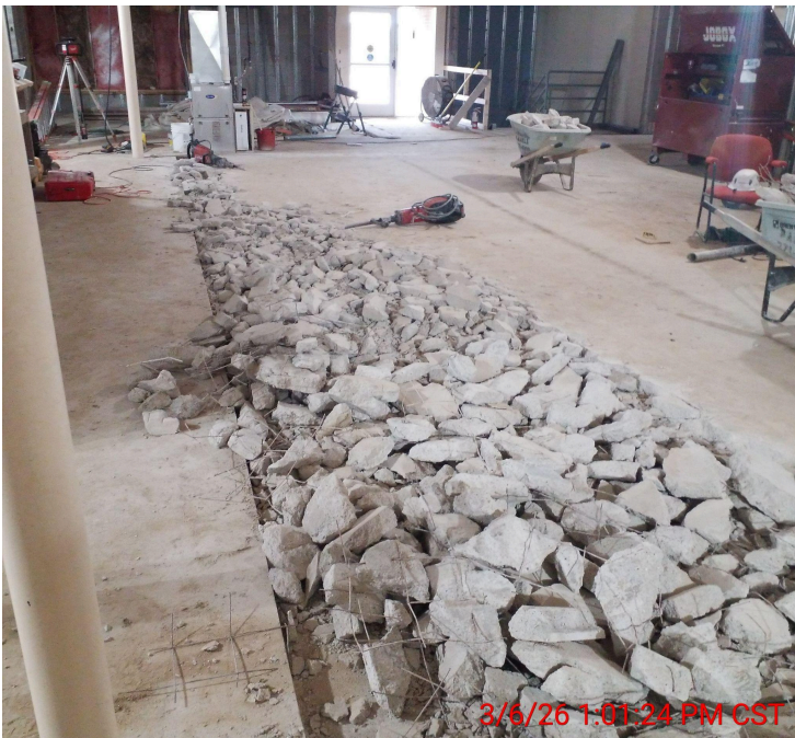
Main level looking W at former front entrance: removal of concrete for opening to lower level
